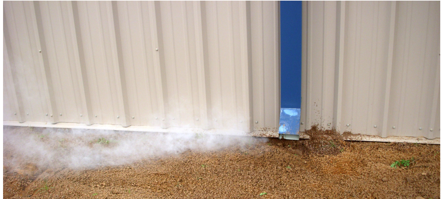
This testing image shows synthetic smoke coming out at the base of the building where the walls meet the foundation.
